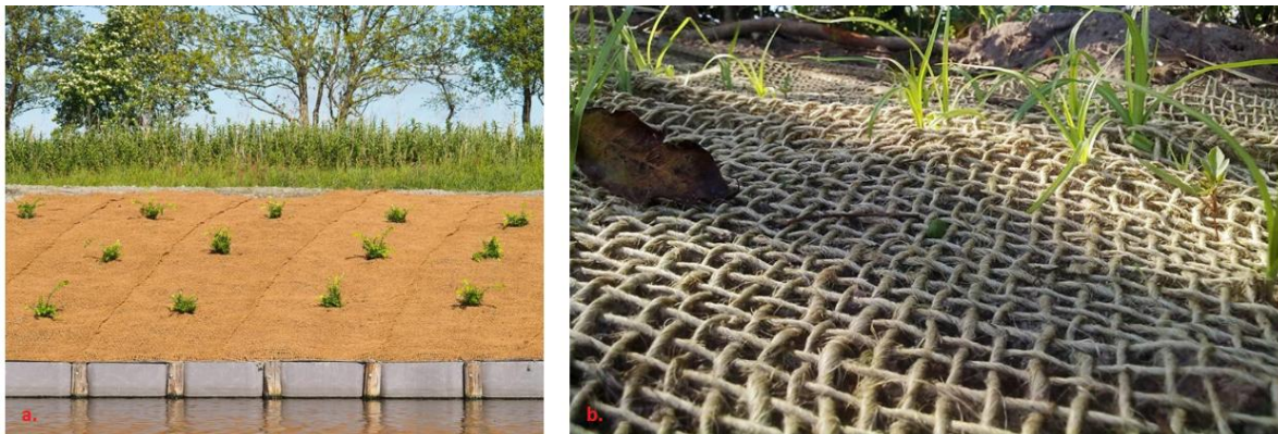
Figure 5: Jute (left) [22] / coconut (right) [23] fiber fabric combined with vegetation planting for shore protection
